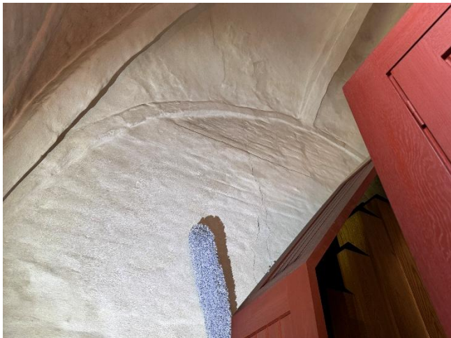
10 – Revner i tårnrum holdes under OBS
